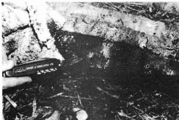
After many hours, the fault is located surrounded by bird nestings.
